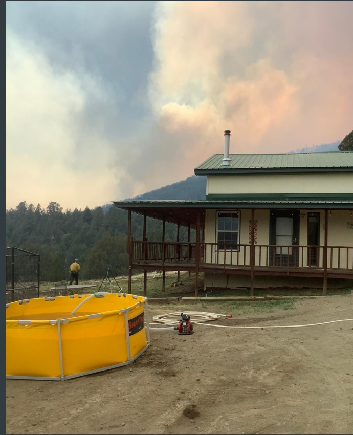
Deploying Sprinkler Systems
